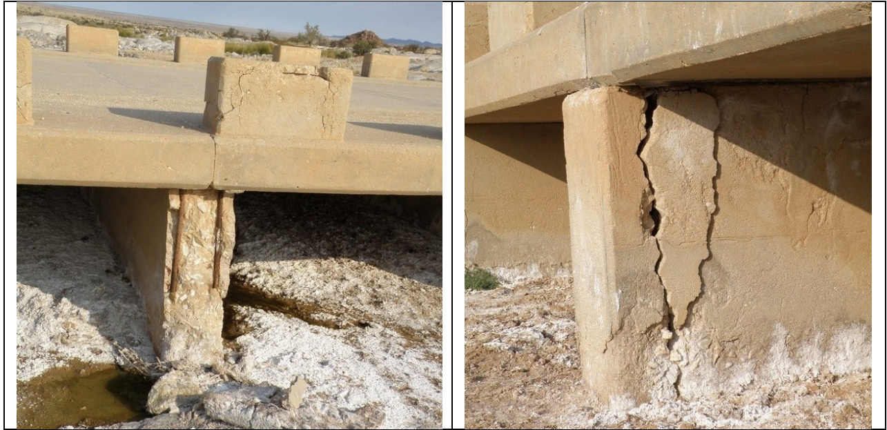
Figure 4. Some defects on Bridge B0090 – Hom River Bridge
