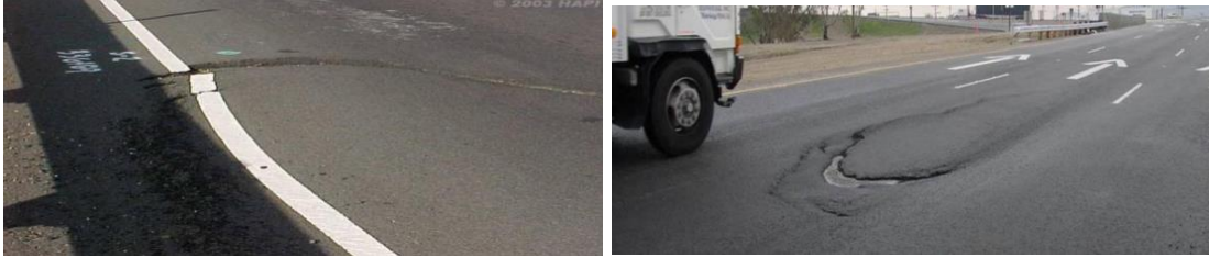
Figure 1: Slippage failure and surface layer delamination of pavement surfaces [2;3]
