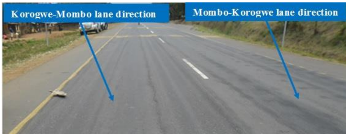
FIG. 6 Rutting on Korogwe-Mombo Section after Two Years of Heavy Trafficking
