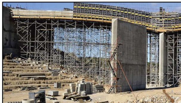
Figure 7: A deteriorating bridge under rehabilitation (Van, 2010)
