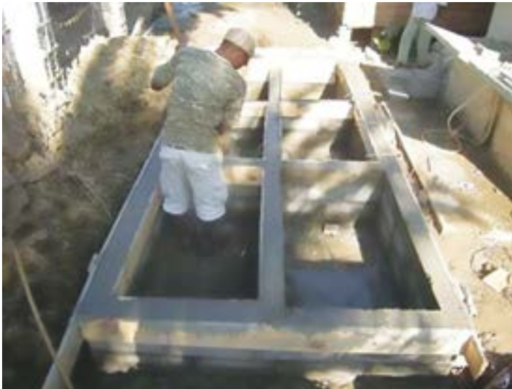
Figure 10.14: A constructed wetland with 3 parallel cells (Hamel, 2011)
