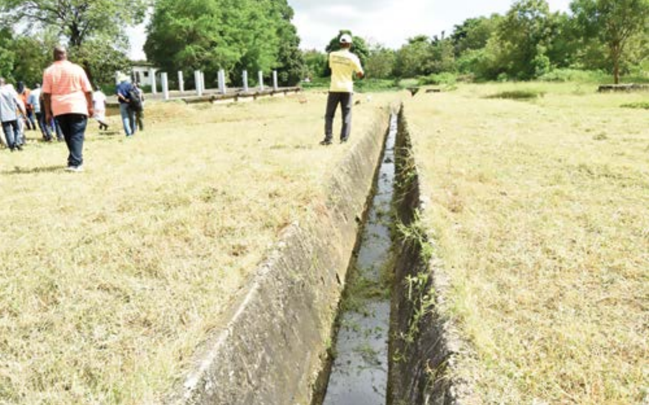
Figure 2.1: Stormwater bypassing the Kipevu wastewater treatment plant in Mombasa draining directly into the Indian Ocean.
