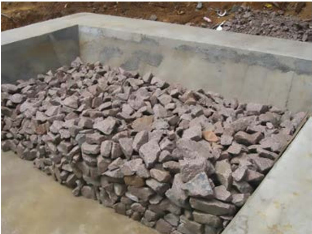
Figure 7.6: Typical clean stones used for inlet and outlet zones (50 - 100 mm) (Credit: Njau et al. , 2010)
