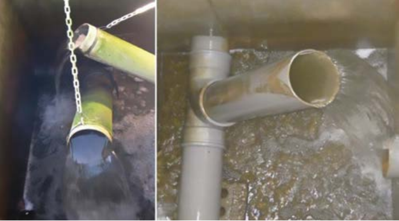
Figure 6.8: Wastewater level maintenance. Left: Outflow pipes hanging on a chain at CW Waikeria, New Zealand. Right: Swiveling elbow at CW Bouvron, France (Photo: Jan Vymazal).
