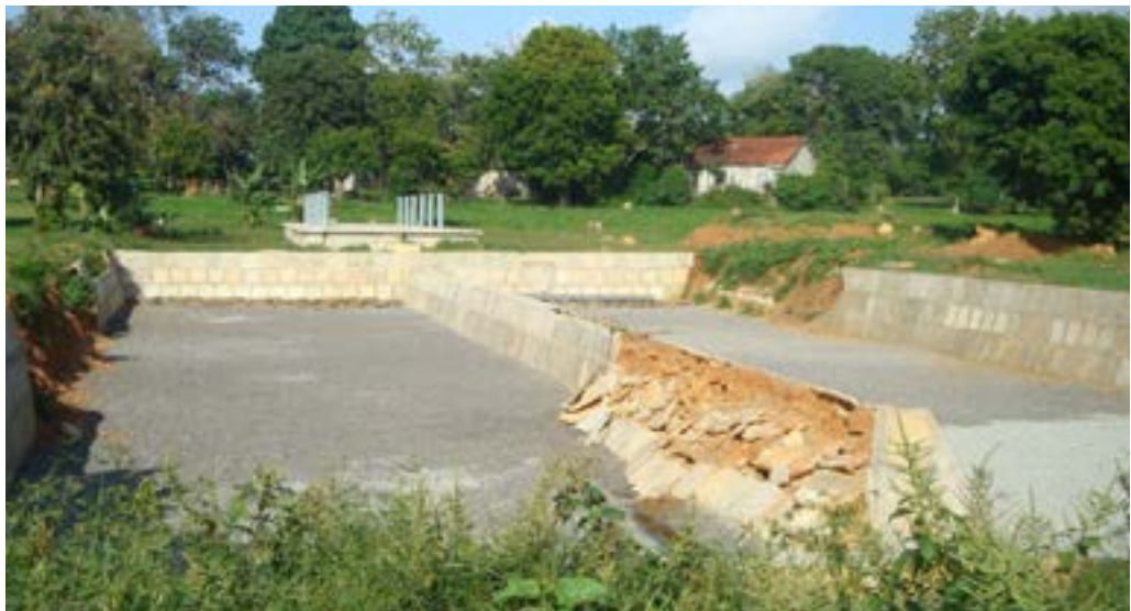
Figure 7.4: Collapsed embankment due to structural instability (Credit: Njau et al. , 2010)
