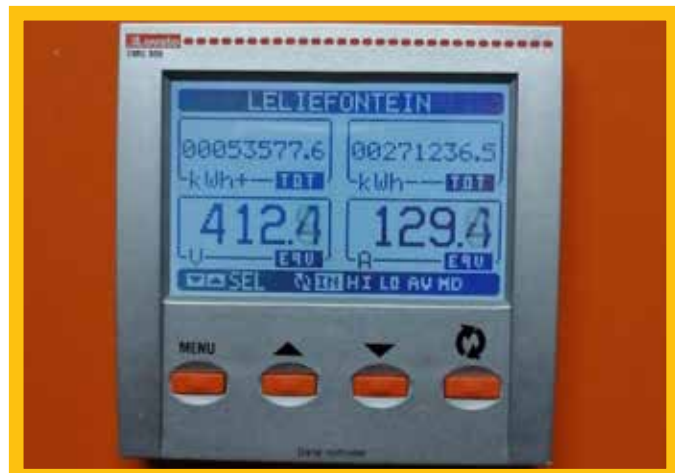
FIGURE 8: Bi-directional power meter at Leliefontein PAT
