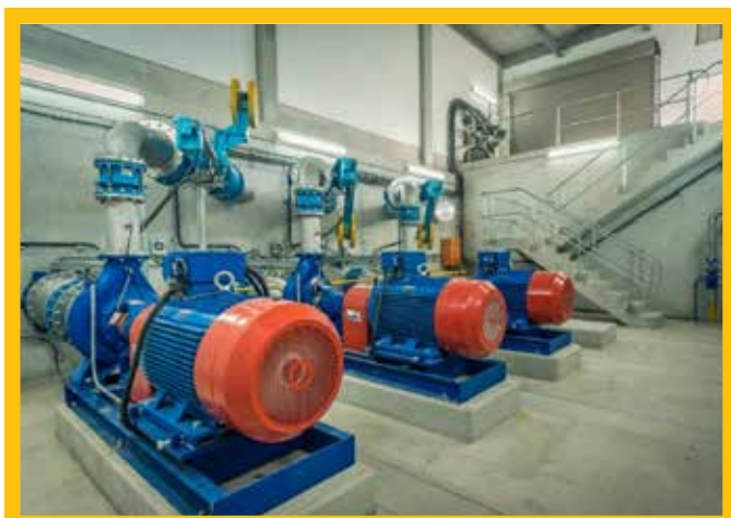
FIGURE 11: Leliefontein Pump-As-Turbines installed, with space for future unit in background
