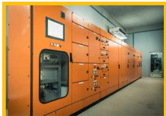
FIGURE 10: Leliefontein PAT Motor Control Centre
