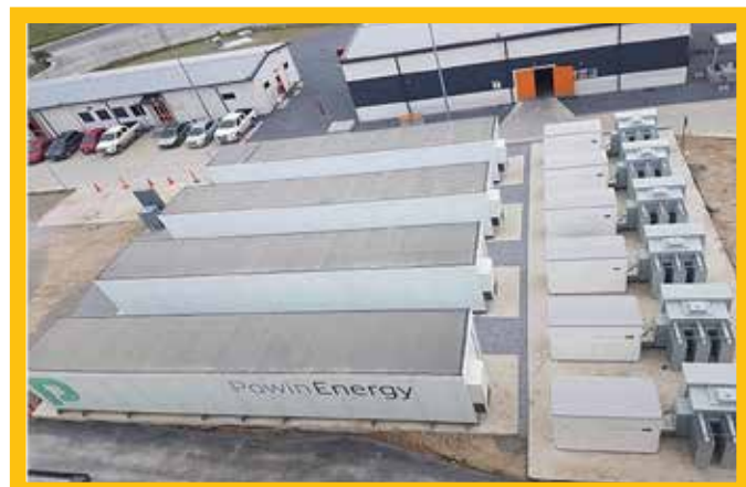
FIGURE 3: 10 MW Battery Installation, Texas US 19
