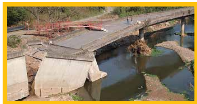
FIGURE 1: The collapsed eastern abutment and end span of the Seaward Road bridge over the Umhlatuzana River
