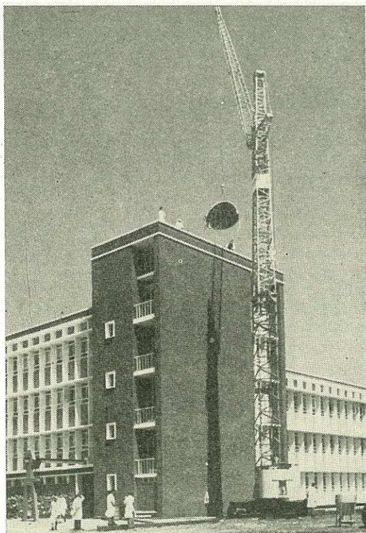
A dome for sun-energy measurement being hoisted on to the roof of the main building of the National Physical Research Laboratory.
