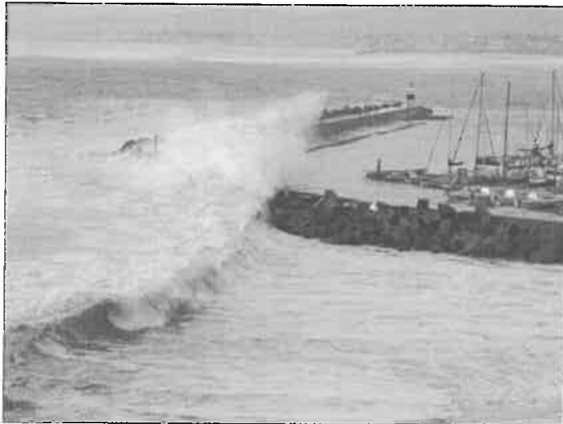
Figure 5: SA example of breakwater barely coping with storm waves at present water levels (Photo: A Theron)
