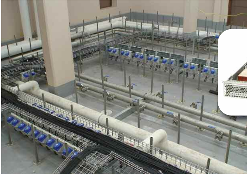
Recently installed chilled-water infrastructure
