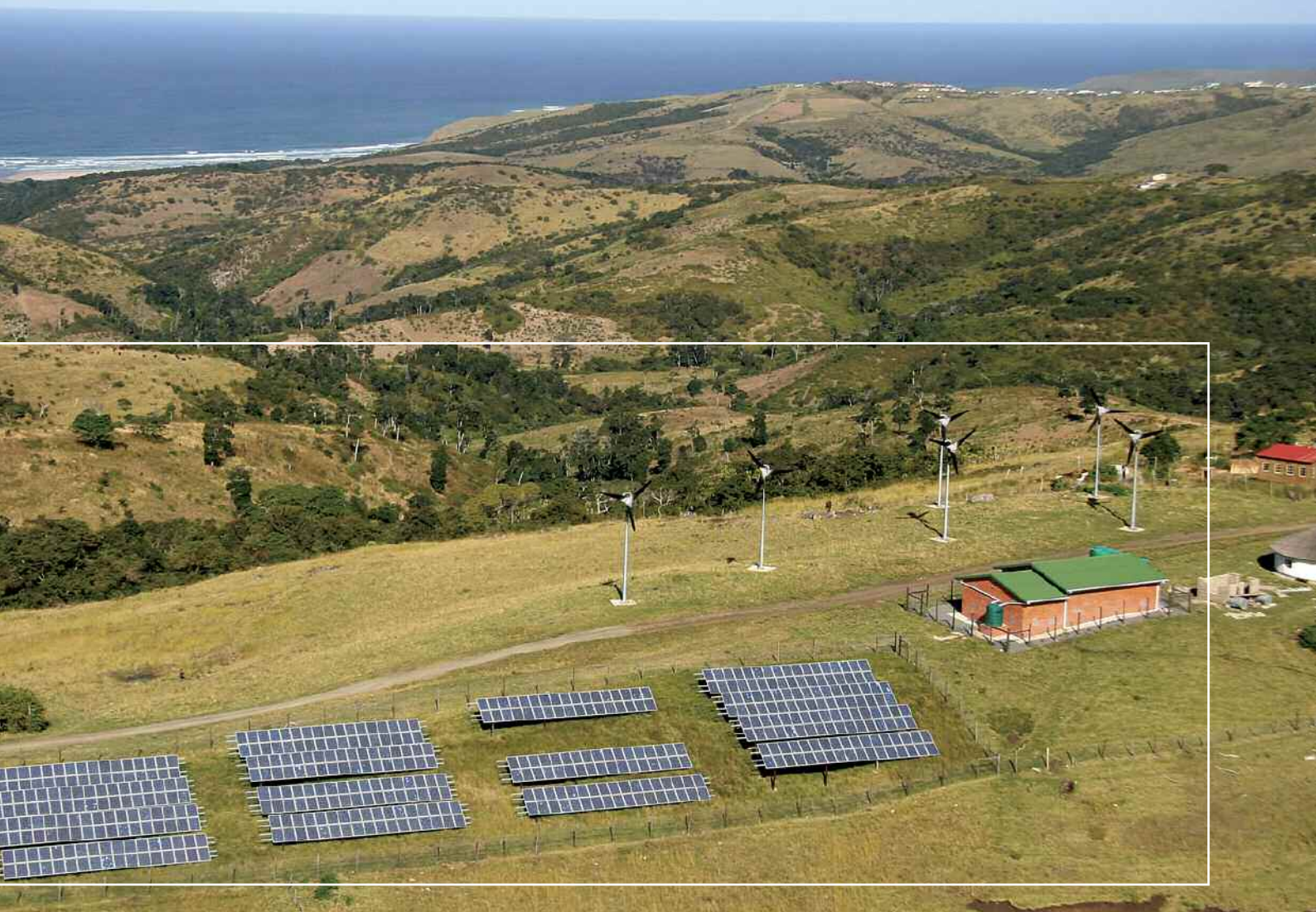
510 solar panels, each with a peak output of 0.113 kW, were erected at a site within the OR Tambo Lucingweni Village
