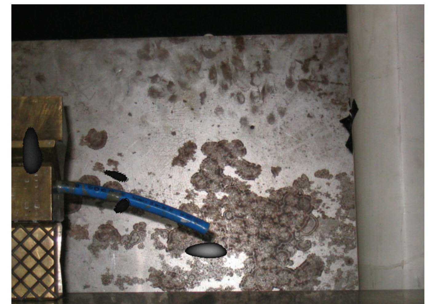
SF 6 gas appearing
