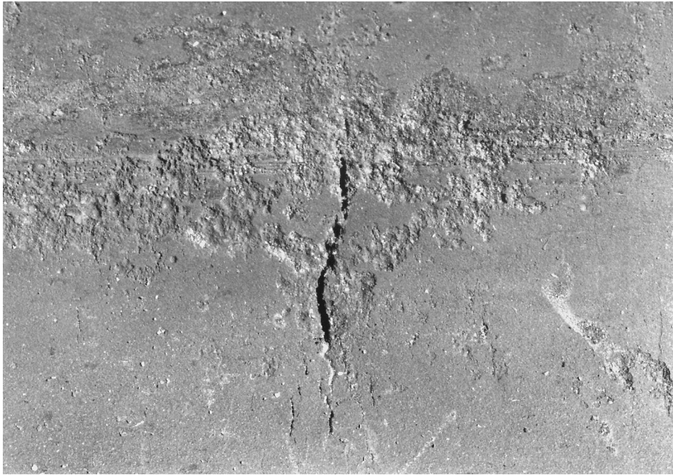
Fig. 6. Close up view of the crack at the point of major leakage.
