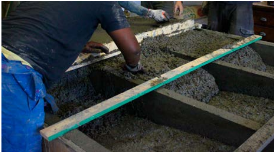
Hand-mixing and casting of a 5-meter unreinforced "nonCrete" funicular floor. Re-usable timber formwork is used in the casting of the floor. Undertaken in partnership with the Block Research Group, ETH Zurich 2022.
