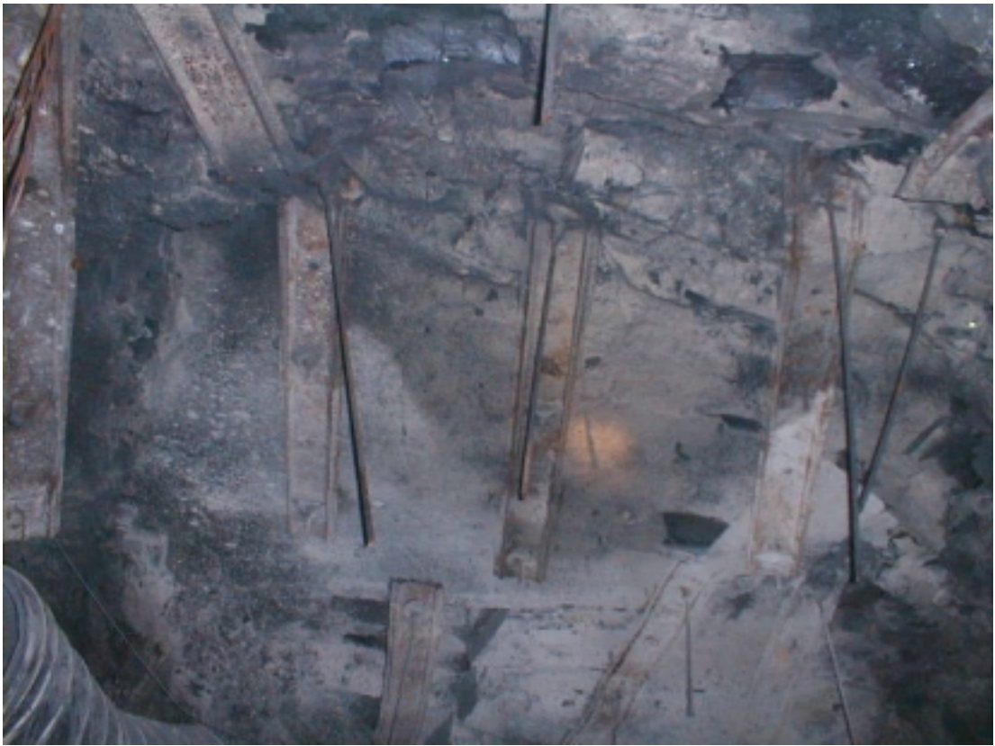
FIGURE 2.4 SOUTH AFRICAN CABLEBOLTS IN-SITU
