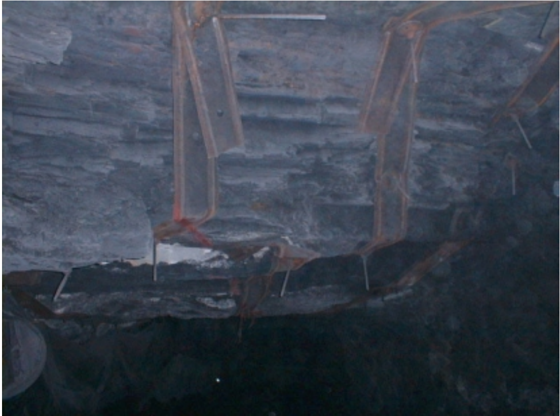
FIGURE 2.5 SOUTH AFRICAN CABLEBOLTS IN-SITU
