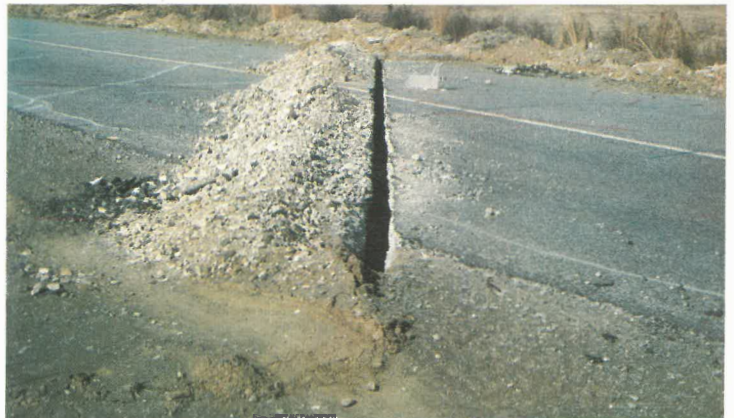
Compressive damage (top) proved to be the worst form of damage to the tarred road as a result of undermining by a total extraction panel. As a preventative measure, stress relieved slots were cut across the tarred road (middle) and after undermining, were repaired with infill and tar surfacing (bottom).
