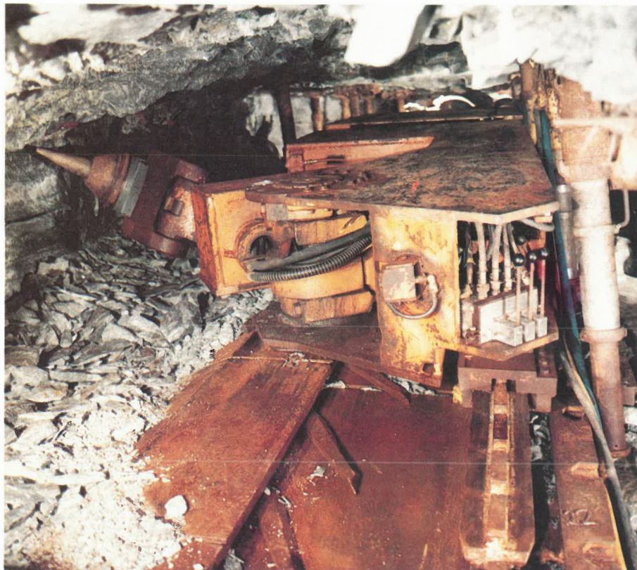
The new prototype impact mining system installed underground at Doornfontein gold mine. It consists of an impact ripping machine which is mounted on a reciprocating flight conveyor and which mines while moving in a down-dip direction. The rock is broken out and loaded onto the conveyor by the hammer manipulation. The machine is currently powered by an emulsion powerpack attached to the back of the machine frame. However, it is envisaged that in future the machine will be powered by water, ideally from a hydro-power system.
