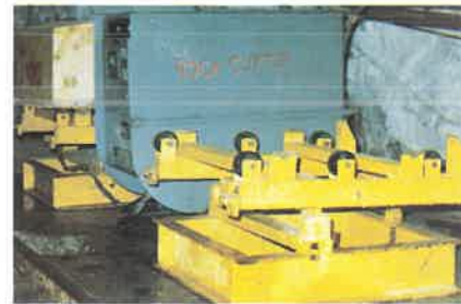
Loco Battery Charging Set
