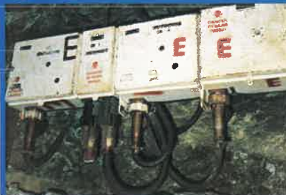
Gully Box Control and Protection Set
