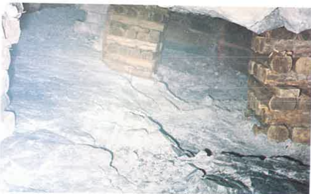
Rough footwall resulting from the absence of favourable parting planes in a stope mined by blasting. This footwall was negotiated by a reciprocating flight conveyor.
