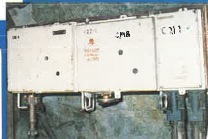
Gully Box Control and Protection Set
