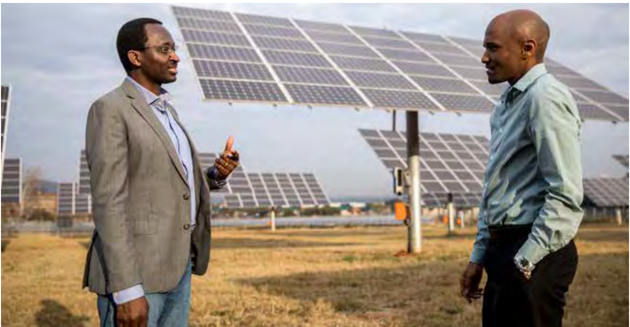
CSIR principal engineer Crescent Mushwana, who leads research into the planning and operation of energy systems and Dominic Milazi, who heads CSIR research into energy policy, at the solar photovoltaic plant on the CSIR's Pretoria campus.
