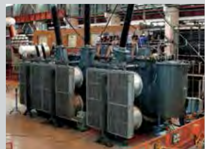
The design of power transformers has been improved.
