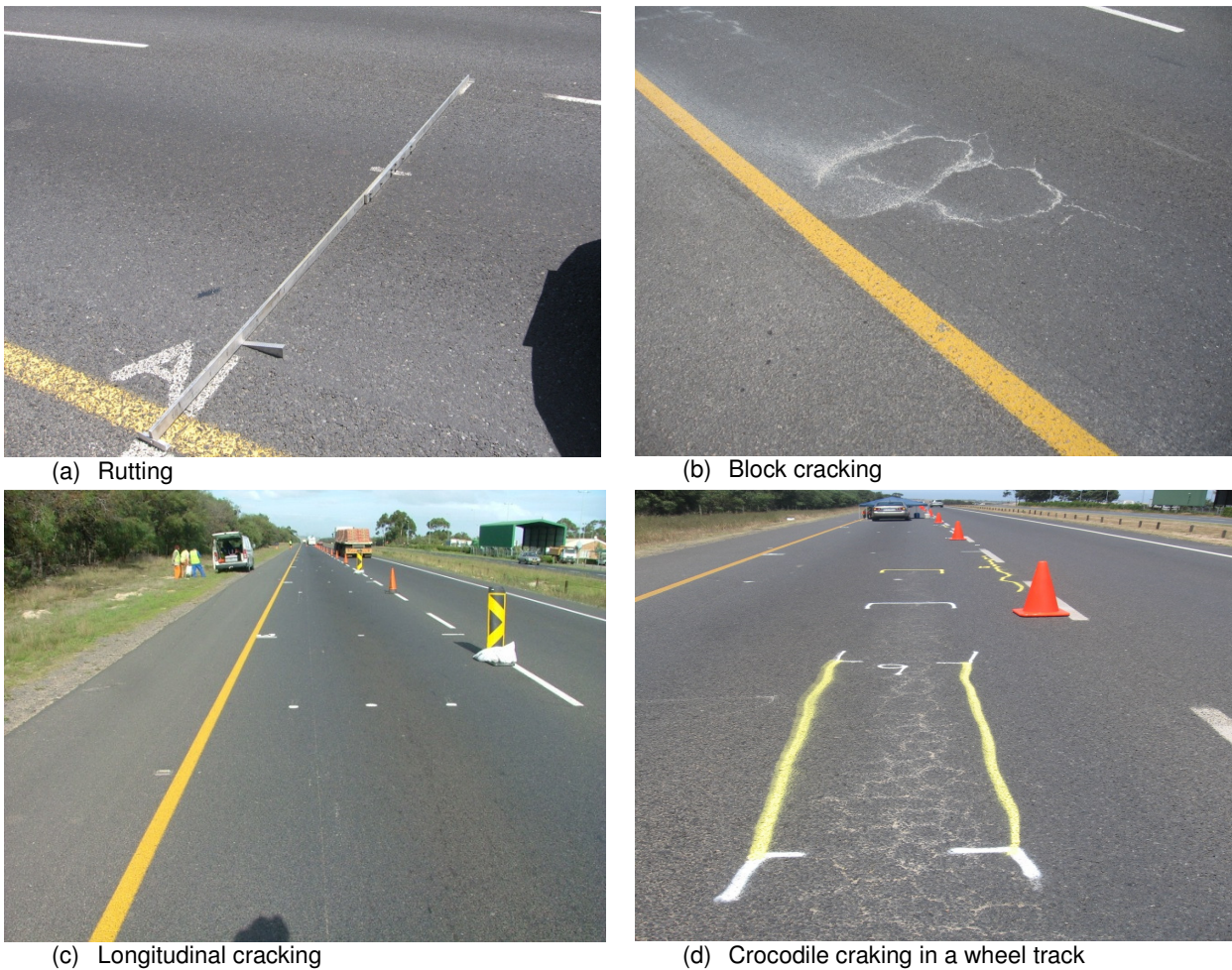
Figure 2 - Various distresses observed on some sites
