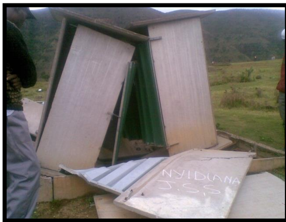
Figure 1 Dysfunctional school toilet facilities
