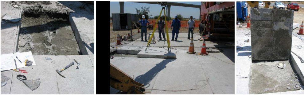
Figure 9. Investigation of void under the slab in Section 2
